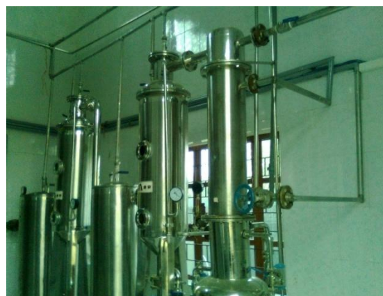
NanoVast water treatment system
